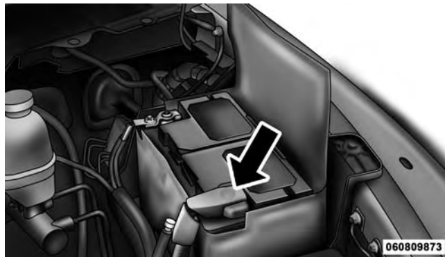
Positive Battery Post
